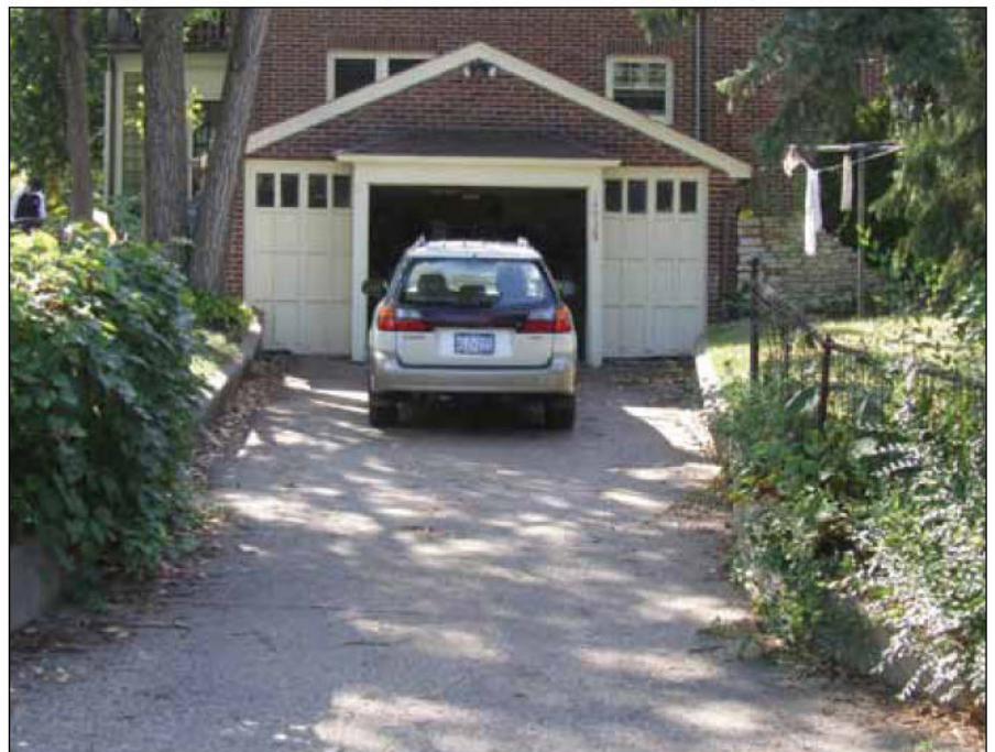
» The original garage was pretty much just tacked onto the house. It didn’t have frost footings. Once torn down, the homeowners cleaned the brick for reuse on the house where brick had been removed during the new garage construction.
